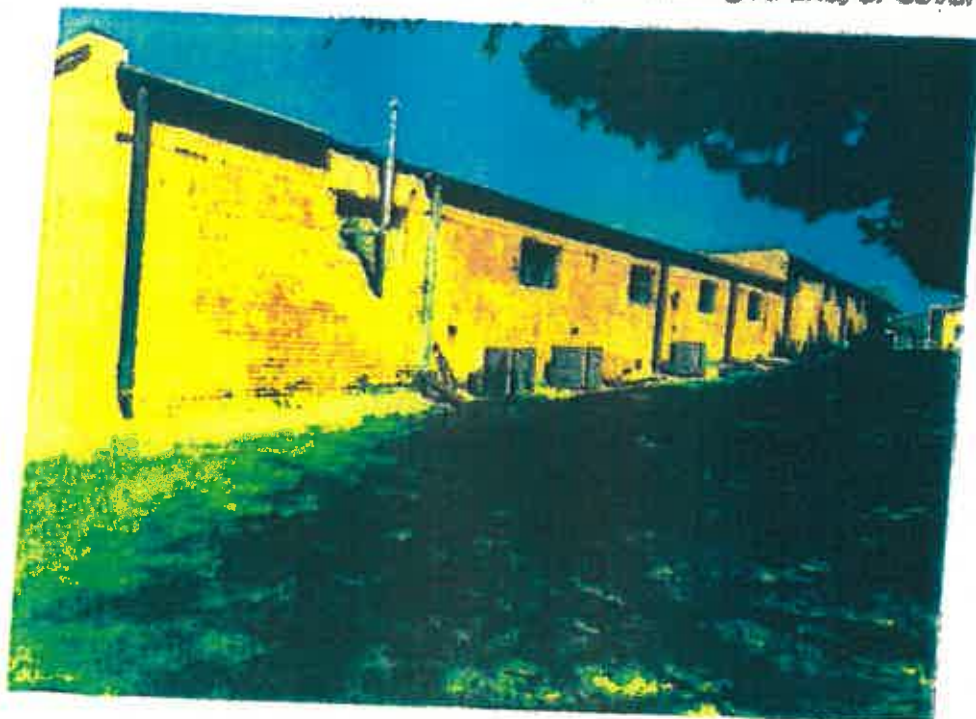
Historic photo depicting what is believed to be the structure at 170 Cleveland Street. The cornice seen here may have been damaged and/or covered .
